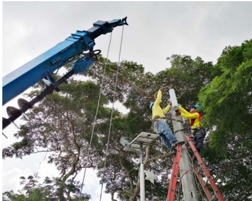
Two (2) members of the Globe network team improve its existing facilities in Bohol to boost connectivity in the province
