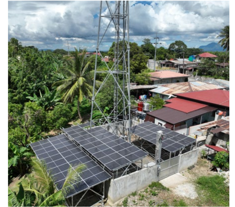
Shifting to renewable energy, such as this cell site in Batangas City, is one of the key strategies of Globe to reduce its GHG emissions.
